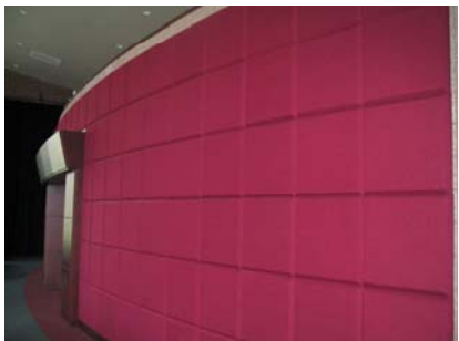
Absorption panels on the rear wall of a performing arts theater
